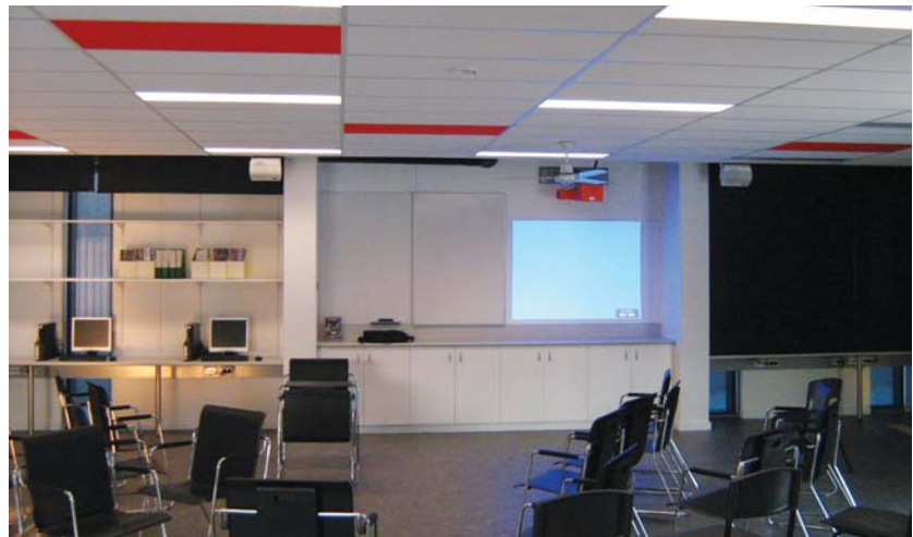
Installation into Science Lounge showing Sanyo PLCXE50 not protruding far from the wall along with 50W self powered speakers on either side
