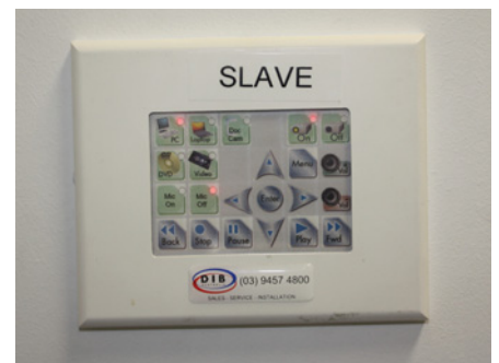
A Joey Lite control panel is installed in each room
