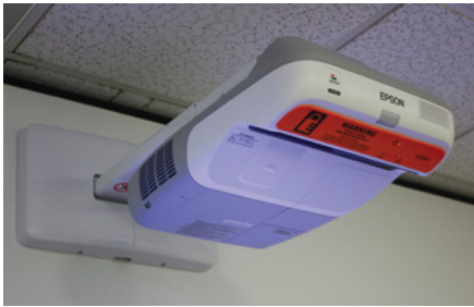
Epson EB-450We widescreen ultra short throw projectors are installed in each of the two rooms of the collaborative learning space
